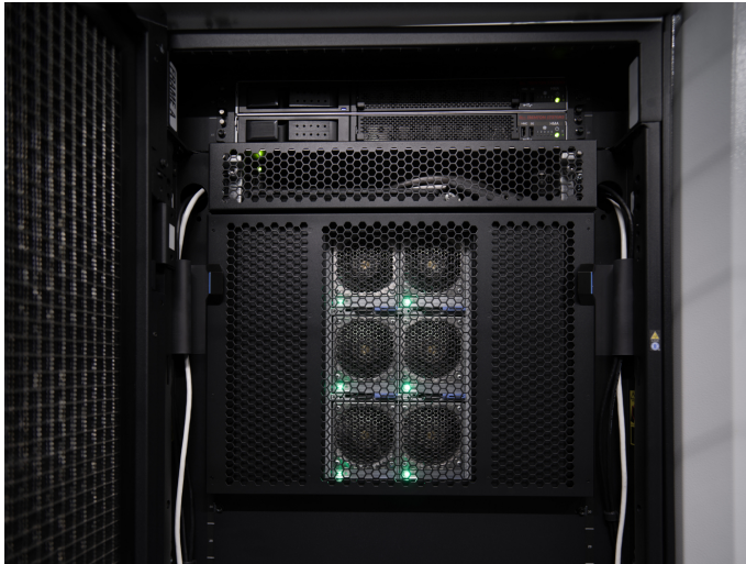
AI-Supercomputer von PHOENIQS in uptownBasel in Arlesheim (BL).
