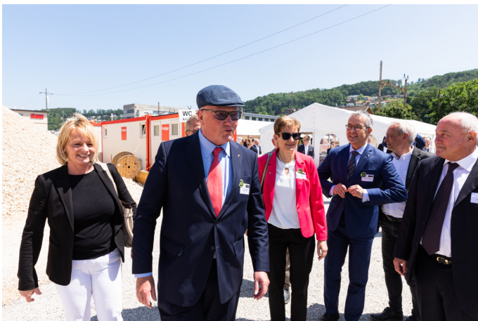
The invited guests on their way to the construction site for the official laying of the foundation stone (from left to right): Elisabeth Schneider-Schneiter, Dr Thomas Staehelin, Dr Sabine Pegoraro, Thomas Weber, Daniel Bürgin and Karl Gun.
